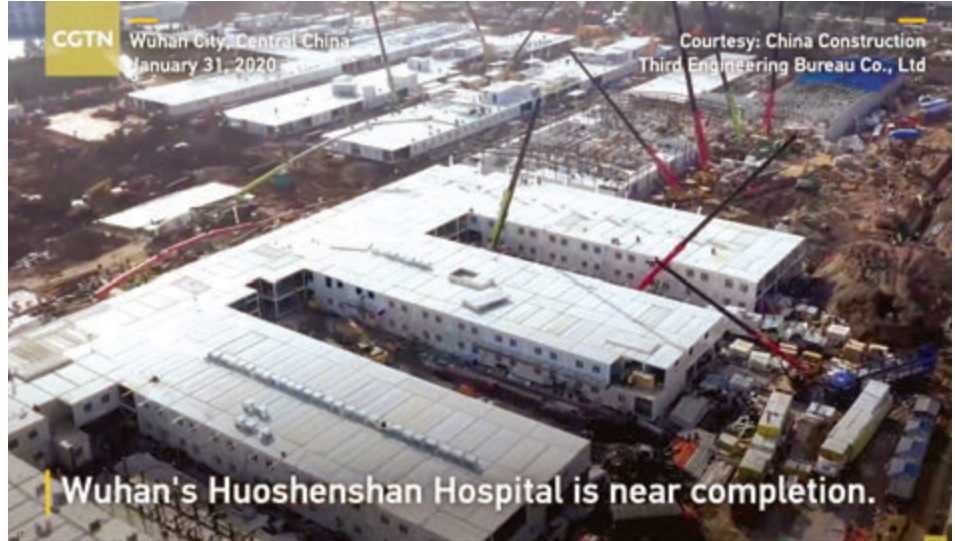
Construction of the thousand-bed Huoshenshan emergency field hospital for COVID-19 patients was begun on Jan. 23 and completed on Feb. 2, with thousands of workers working around the clock. This photo was taken on Jan 31. Leishenshan Hospital, built with the same design, was finished on Feb. 8.
